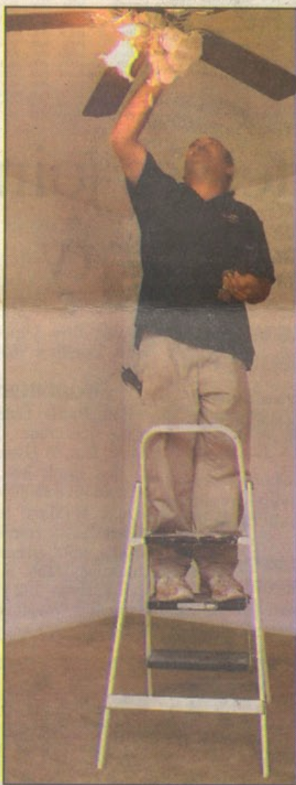
Frank Amador checks a ceiling fan in an apartment undergoing renovations at Madison Court Apartments.
